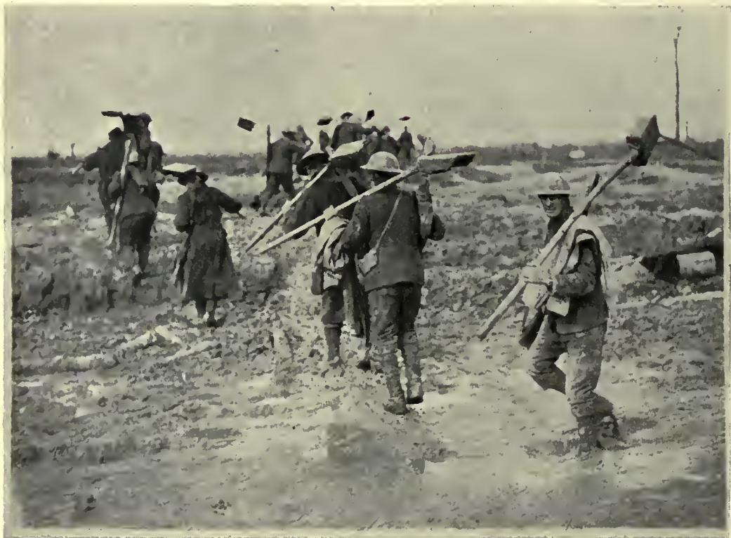
OFF TO CLEAR UP THE FLOODED ROADS.
