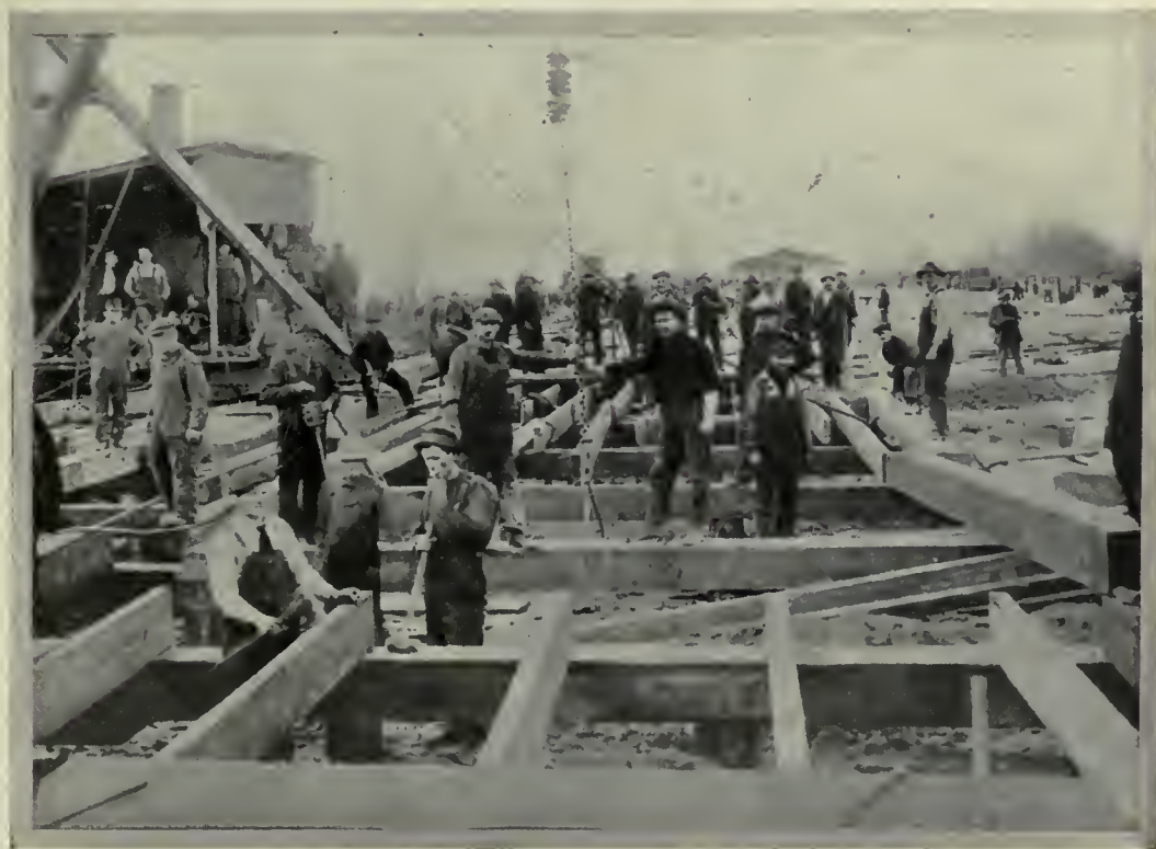
LAYING TIMBERS FOR A NEW AMERICAN DOCK AT A PORT IN FRANCE.
